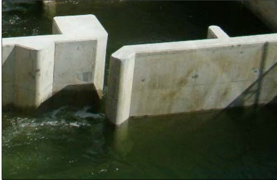
Figure 16. New vertical slot weirs at John Day North Ladder feature rounded (minimum 4-inch radius) edges. Rounded edges help lamprey navigate high velocity and/or high turbulence fishway features.
