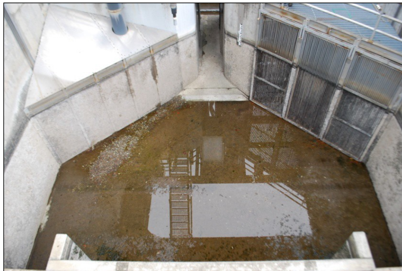
Figure 10. Dewatered count station at The Dalles Dam East Fish Ladder, facing upstream. Picket leads (at right) guide fish to the count slot (left). Picket lead panels have been elevated off the fishway floor by 1 to 1.5 inches to offer lamprey an alternative passage route.
