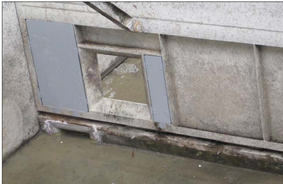
Figure 15. Newly installed lamprey orifice in the MCN Oregon Shore Fish Ladder, tilting weir stem wall (lower left). Additionally, steel plating was installed around the elevated orifices to provide attachment surfaces for adult lamprey.
